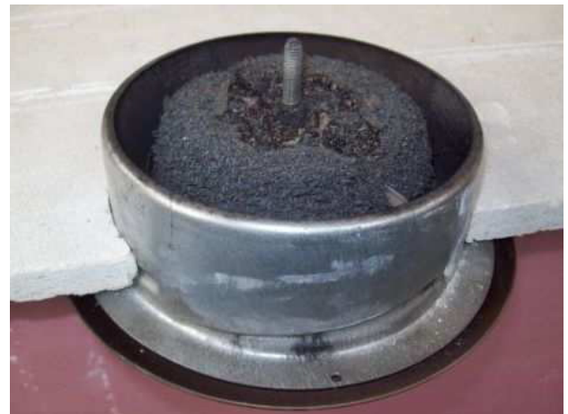
Fire Rated Ceiling Air Valve sealed after a fire
